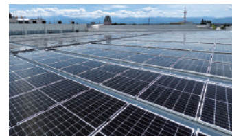
The solar power generation system (installed at our Toyama Plant)
